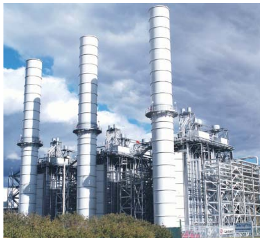
TransAlta's gas-fired cogeneration plant in Sarnia, completed in 2003, is one of the newest generating stations in Ontario.
